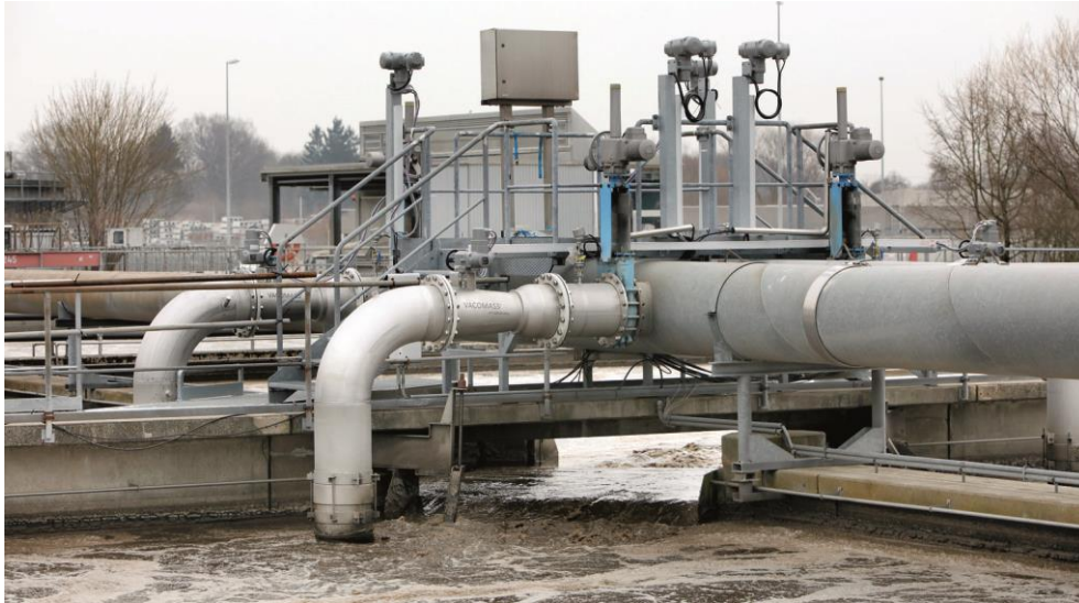
Photo: Wastewater Treatment Plant Ulm-Steinhäule
